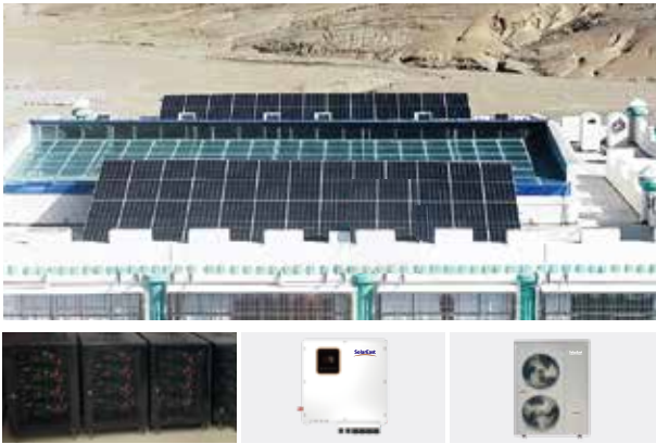
PV+Storage+Thermal project for 17 elementary schools, Tibet
