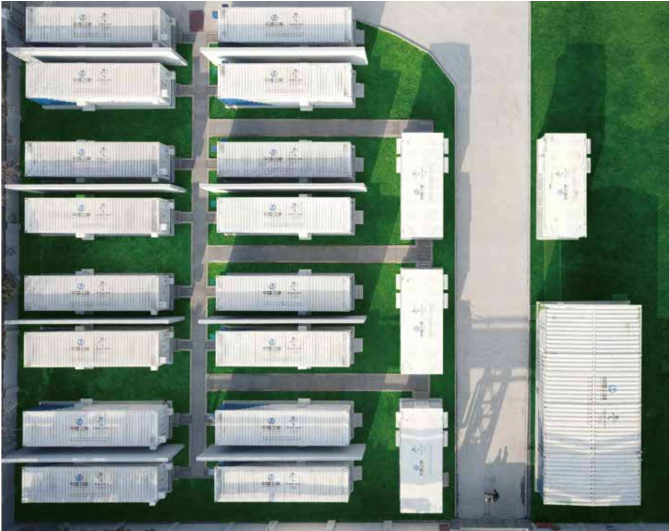
10MW/39MWh Energy Storage Station
