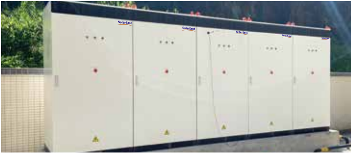
Industrial & Commercial Energy Storage Project, Guangdong
